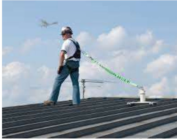
Fig. 4. An example of a fall protection system, when working on roof edge/corner.
